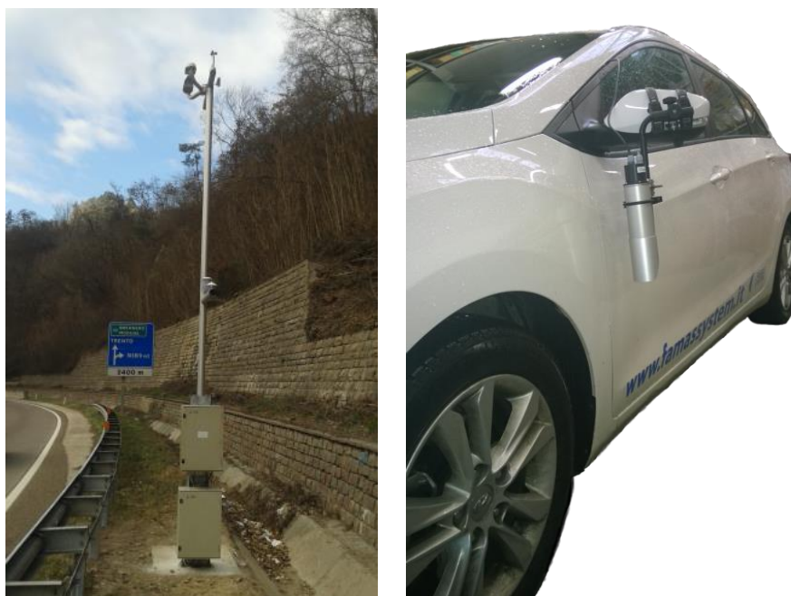
Figure 14: The Civezzano RWIS station (left) and the enhanced mobile RWIS station demonstrator (right).
